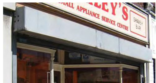
✗✗ Bulky and unsightly roller shutter housing obscures the top of the shopfront
