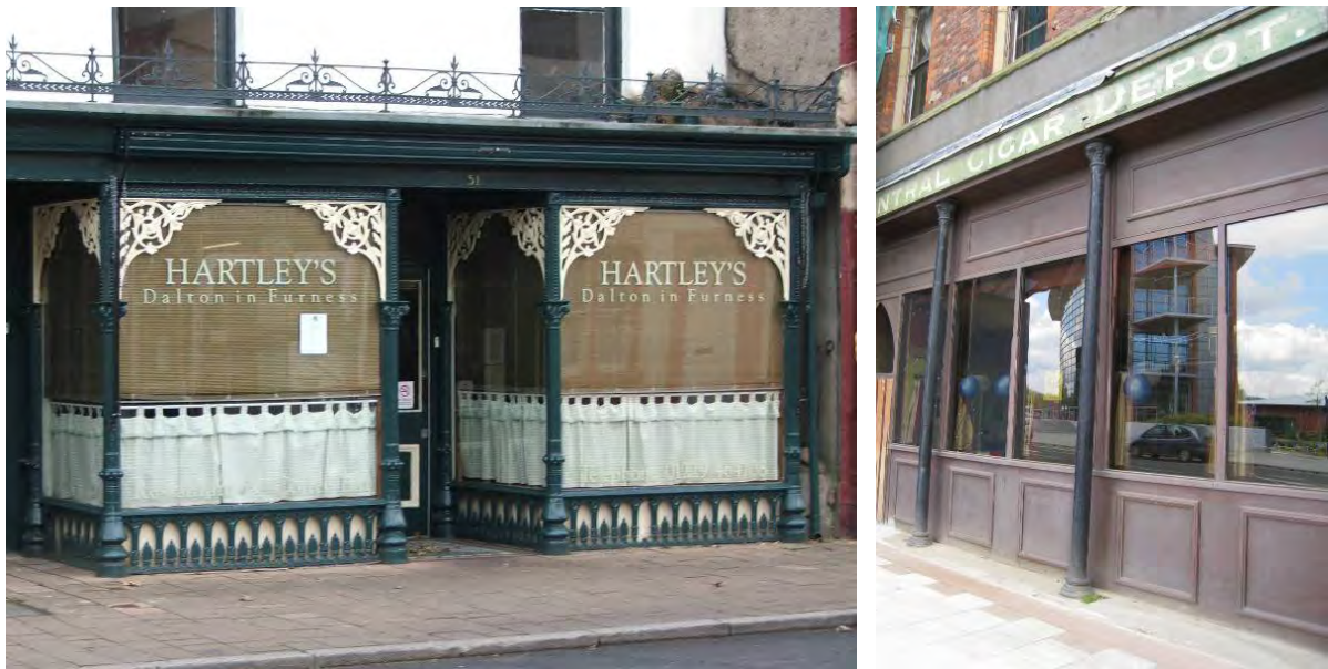
Left: Cast iron shopfront at Dalton-in-Furness with colonettes and fretwork. Right: Cast iron columns at Oxford Chambers, Duke Street, Barrow
